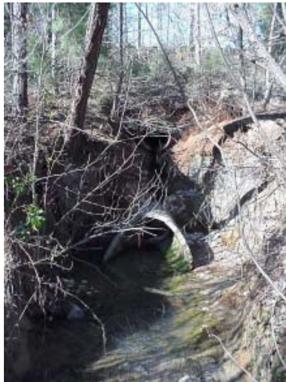
Exhibit D.8 Undercut culvert draining Waverly Place
