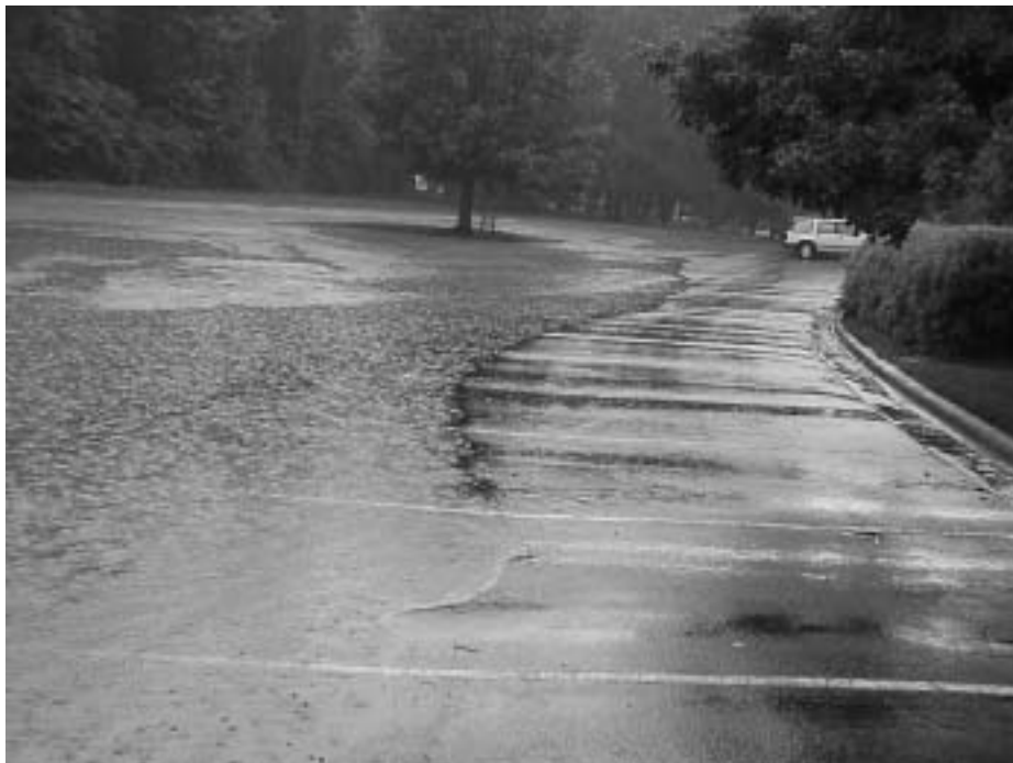
Exhibit D.4 Out of bank flow in Williams Creek floods MacGregor Center parking areas
