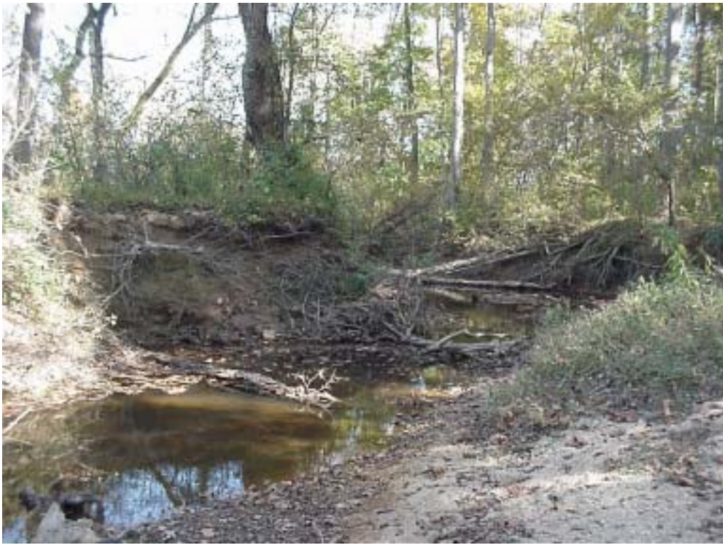
Exhibit 6.1 Bank erosion on Swift Creek upstream of Holly Springs Road
