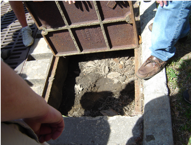
Figure 11-3b Sand Filter Chamber Overdue for Maintenance
