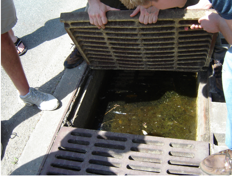
Figure 11-3a Sedimentation Chamber Overdue for Maintenance
