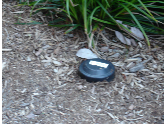
Figure 12-6 Bioretention Cell Clean Out Pipe, Less than the 8" Recommended Height
