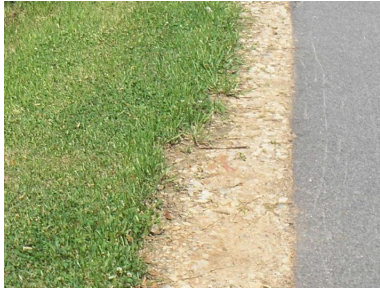
Figure 12-8a Gravel Pretreatment is Clogged with Sediment
