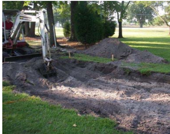
Figure 18-15. Where possible, excavate soil from the sides of the pavement area to minimize subgrade compaction from equipment. Source: NCSU-BAE
