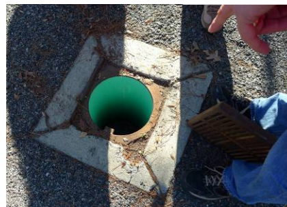
Figure 8-10. An observation well enables inspection of water infiltration.
