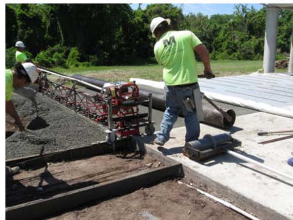
Figure 18-23. Pervious concrete paving lane filled between cured lanes forms a parking lot. Source: NCSU-BAE
