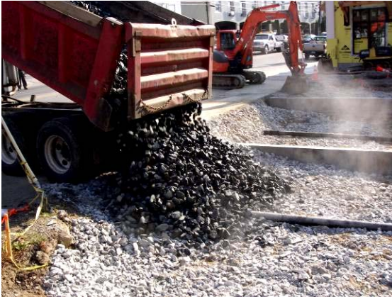
Figure 18-19. A dump truck deposits aggregate directly into excavated area for spreading. Source: NCSU-BAE
