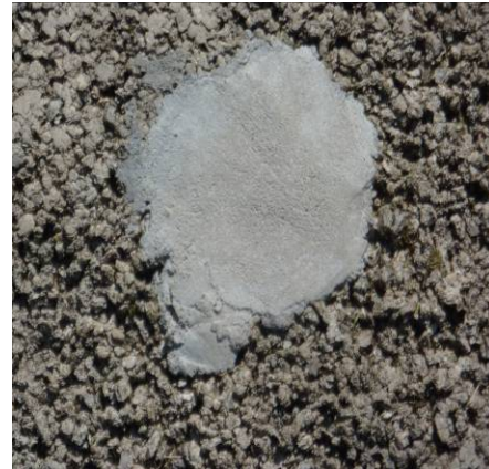
Figure 18-27. Patching areas of permeable pavement with impervious material shall not exceed 5% of the total area.
