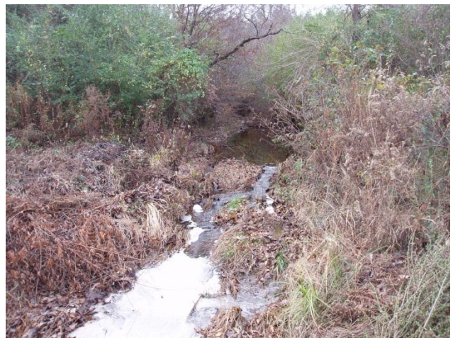
Upstream of structure (headcut located above white foam)
