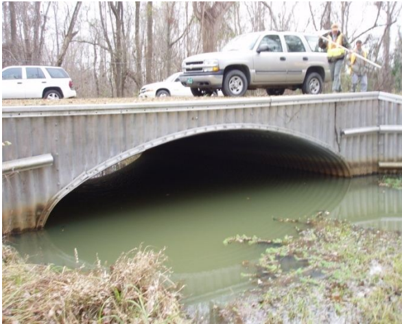
Inlet of structure – no fill against headwall
