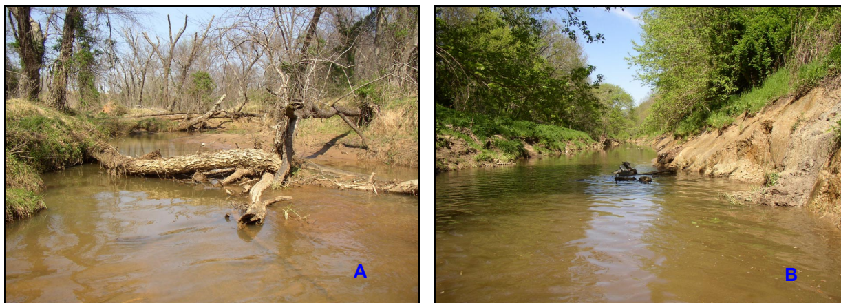
Figure 2. Sandy substrates without riffles, vertical and eroding banks, and sparsely vegetated riparian zone (Picture A). Picture A = Richland Creek, US 1, Wake County, and Picture B = Ellerbe Creek, SR 1709, Durham County.
