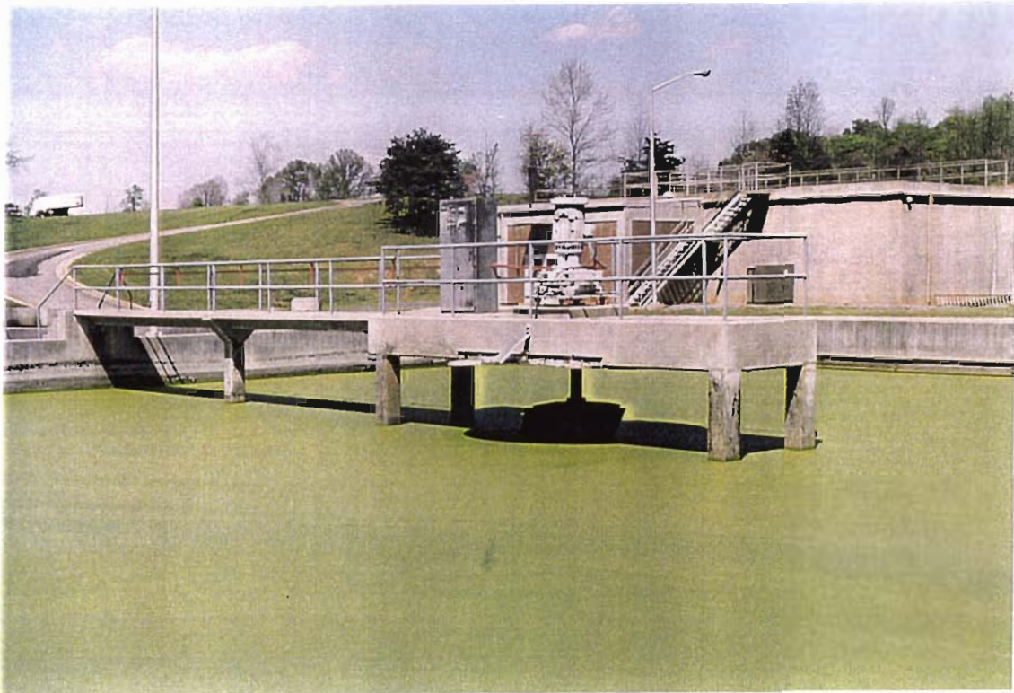
Duckweed in aeration pond of a wastewater treatment plant, Roxboro, Person County
