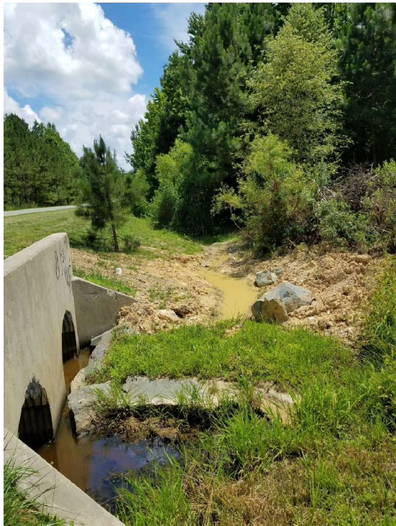
Figure 19: Degraded Buffer and Sediment Excavation (?) on Dry Creek's Long Branch Tributary
