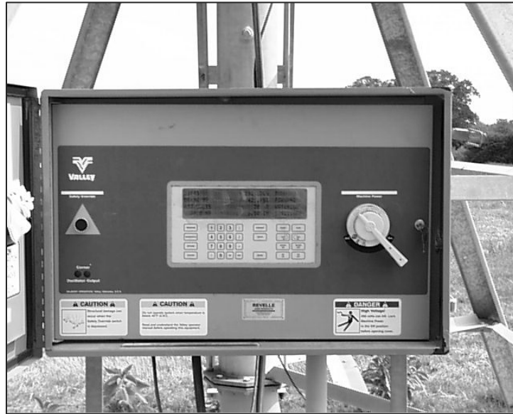
Figure 4-19. Center pivot control panel.
