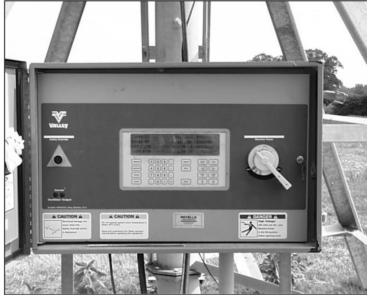
Figure 4-19. Center pivot control panel.
