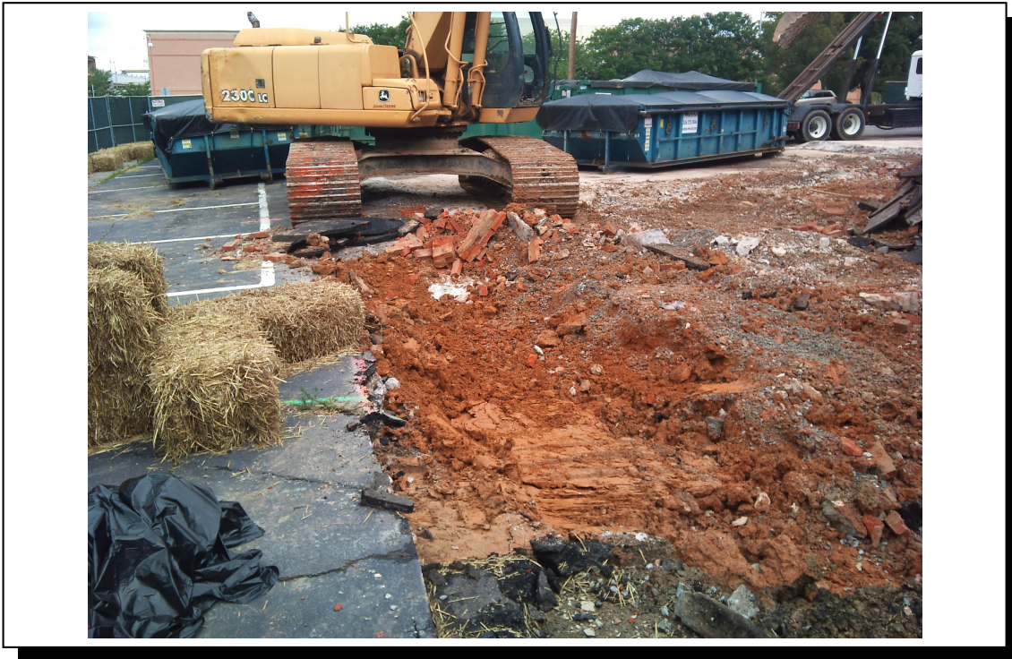
Description: View of brick footing and asphalt placed in roll-off container #380RT.
